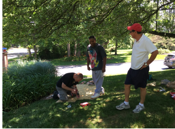
Robert Jones and Jim Dillard help Brandon Boron repair Lakeside and Dockside entrance Signs
